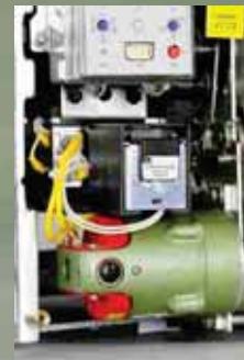
Motor / Remote connection
